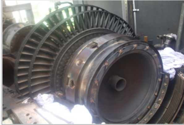
Figure 1: Gas turbine during the operation of its periodic maintenance.
