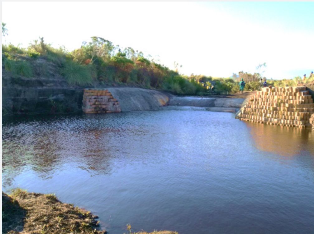
Figure 2: The erosion has been deactivated with the construction of an energy dissipating chute; also preventing further draining of the peatland.
