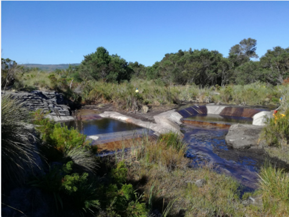
Figure 3: Smaller erosion features were de-activated and the water levels within the peat restored with smaller concrete chute interventions.
