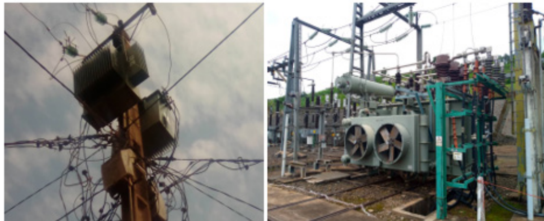
Plate 1: Exposed electricity transmission infrastructure.
