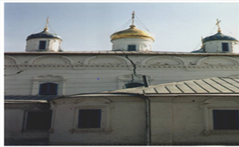
Figure 1: Crack above the window opening of the temple (northern facade).
