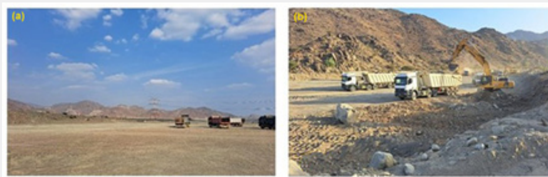
Figure 11: Dredging and trucking of the silt from Ham (Inset a) and Safad reservoir (inset b).
