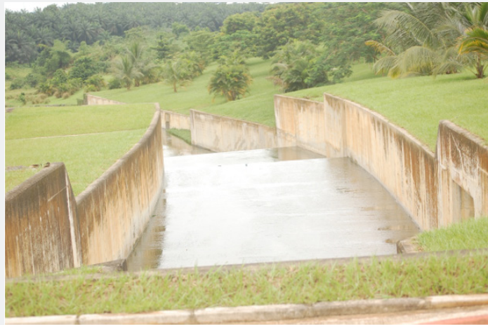
Plate 3: Brook Street rehabilitated gully site with green edges, Uyo urban, Akwa Ibom State, Nigeria.
