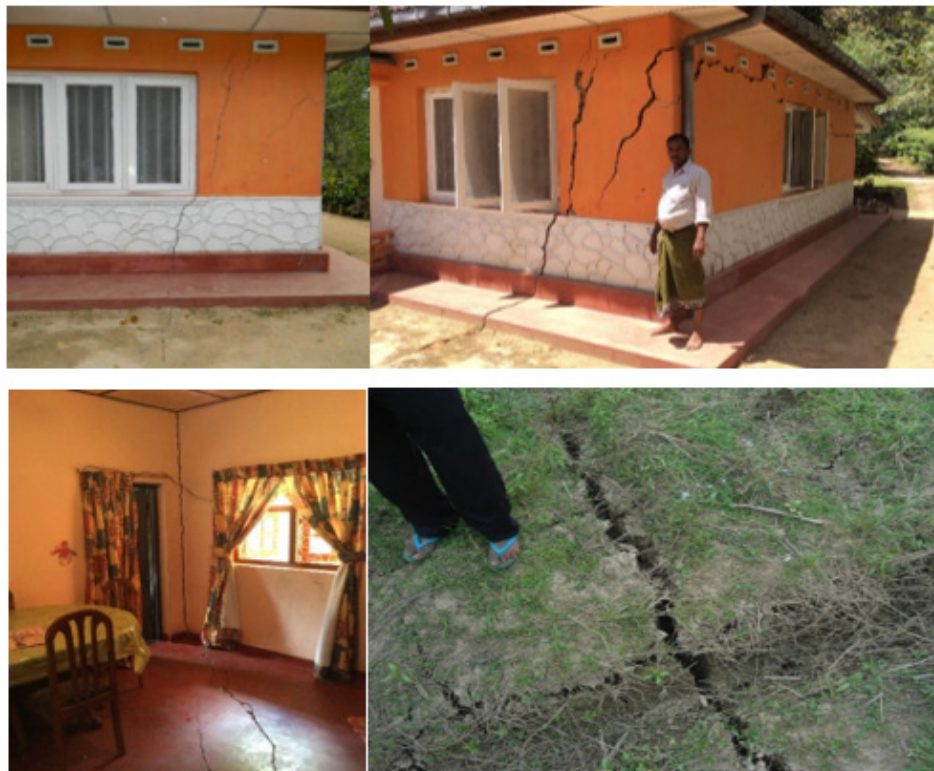
Figure 9: Cracks developed in the soil and houses in the Makulella area in December 2014.
