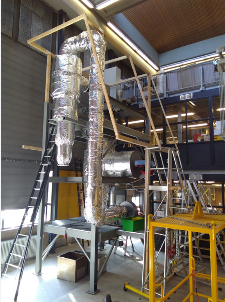
Figure 3: Heat treatment of fines and lights (industrial prototype at 3ton/h).
