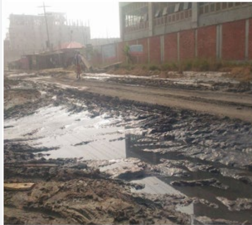
Figure 4: Waterlogging in the internal roads of the industrial area.
