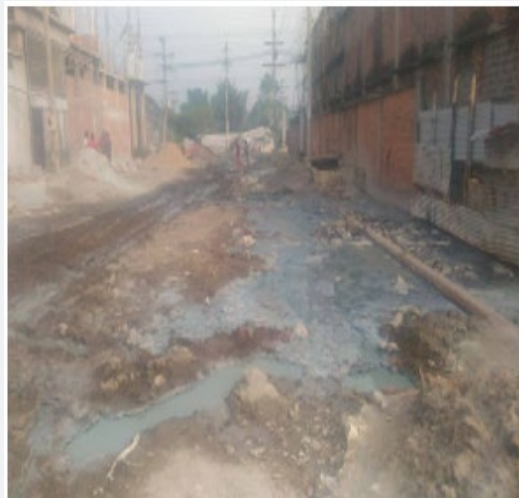
Figure 5: Waterlogging in the internal roads of an industrial area with unbearable malodor.
