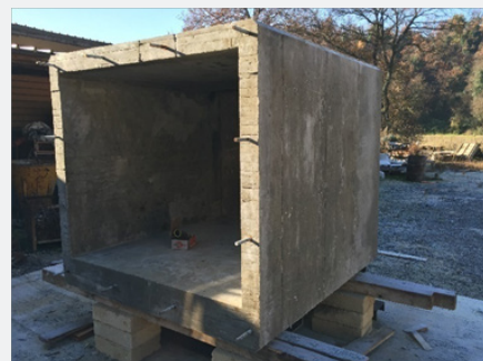
Figure 9: Main body of the APE SR facility.
